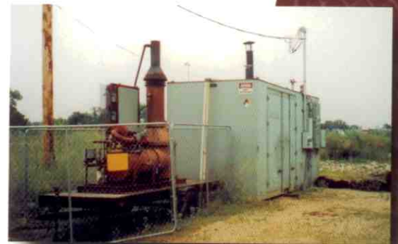
Groundwater Remediation System
