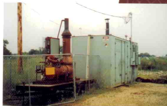
Groundwater Remediation System
