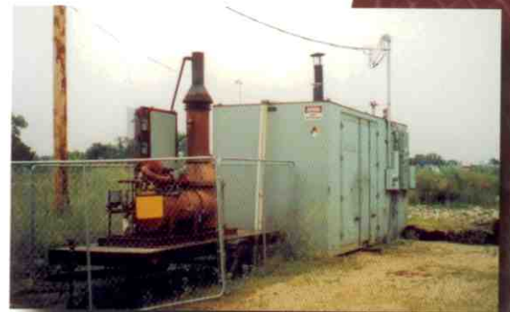
Groundwater Remediation System
